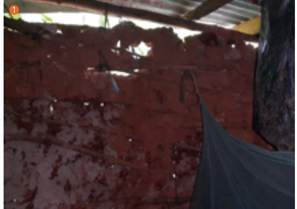
① Mud hut with a hole in the wall
