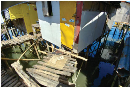
Huts that appear to be on the verge of collapse
